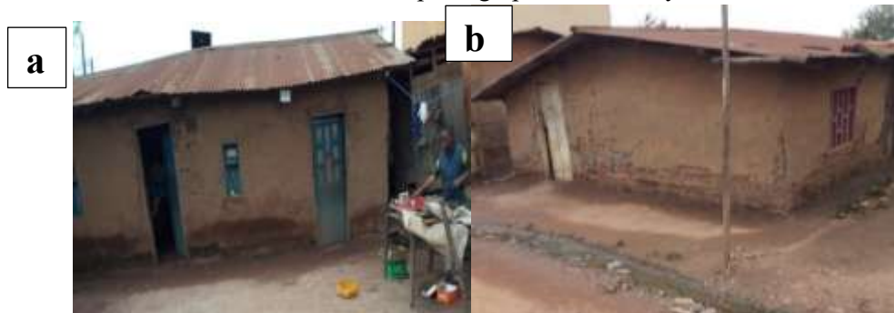
Figure 2. Overview of the subsidence of the buildings which are in a very advanced state of disrepair.
